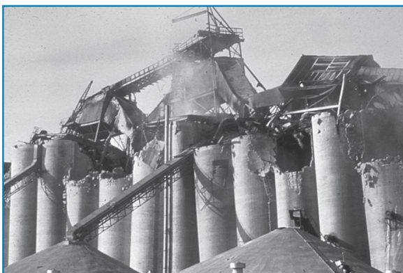
ELIMINATING DISASTERS LIKE THIS REQUIRES CAREFUL CLASSIFICATION OF AREAS AND THE USE OF THE PROPER ELECTRICAL EQUIPMENT.
